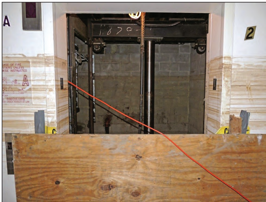
Figure 5-28. Hydraulic elevator in New York City hospital flooded during Hurricane Sandy.
