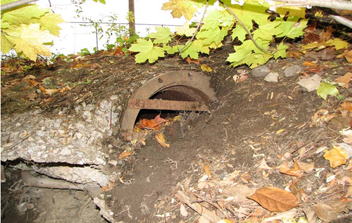
An outfall on Spring Run – abandoned. Do NOT call.
