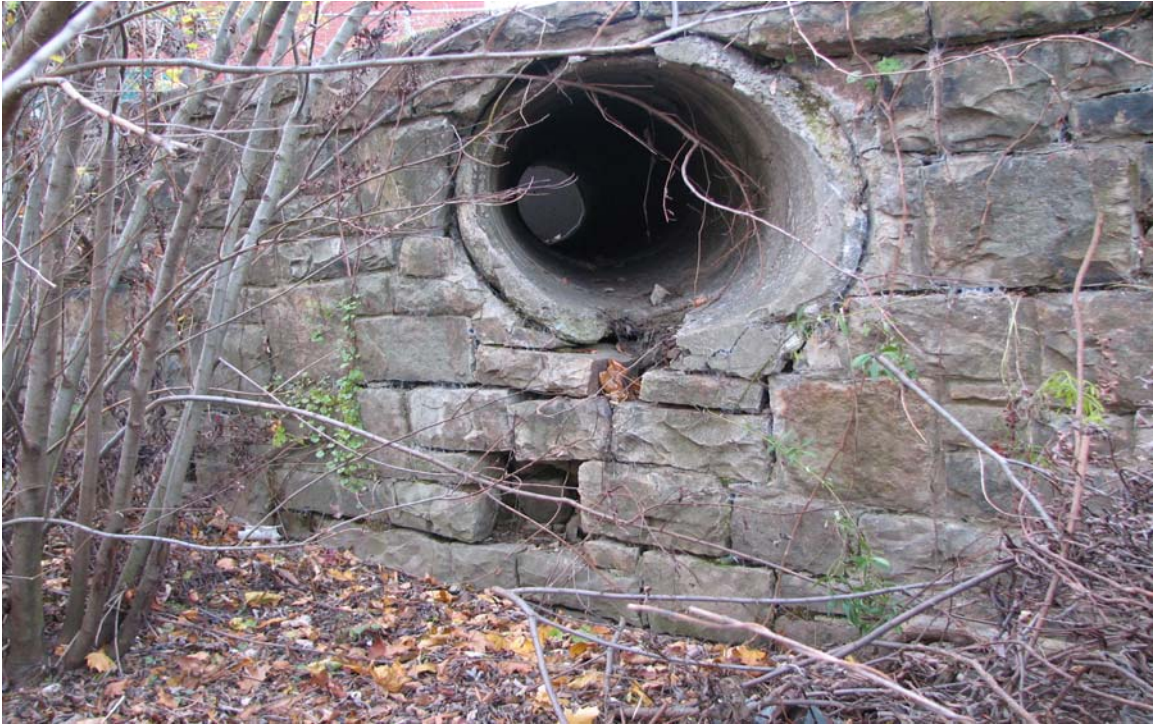
Outfall– scheduled to be repaired (Do NOT Call).
